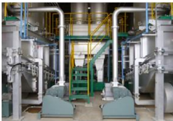
Biomass boiler at Odate Plant
